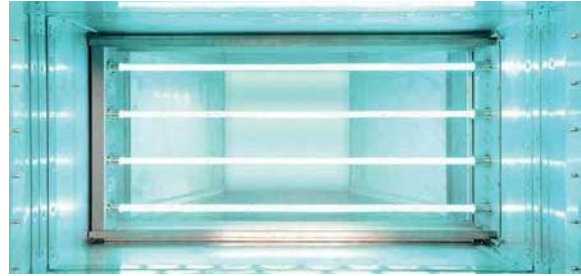
Efficiently integrated UV lamps in an air duct.
